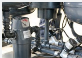
Air Filter - Pic. 4
